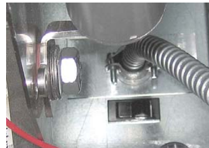
Figure 14 (Rear view of Control Box)
